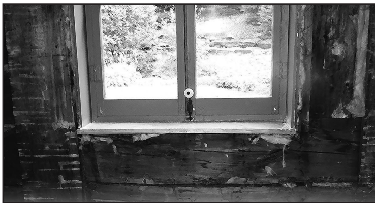
Wall where the 1873 letter to Mrs. Millar was discovered under the plaster. Photo courtesy of Yolande Allard.
