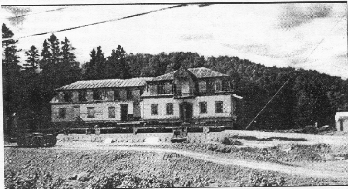
Before workers renovated the LeGrand Hotel they jacked it up to build a foundation.
